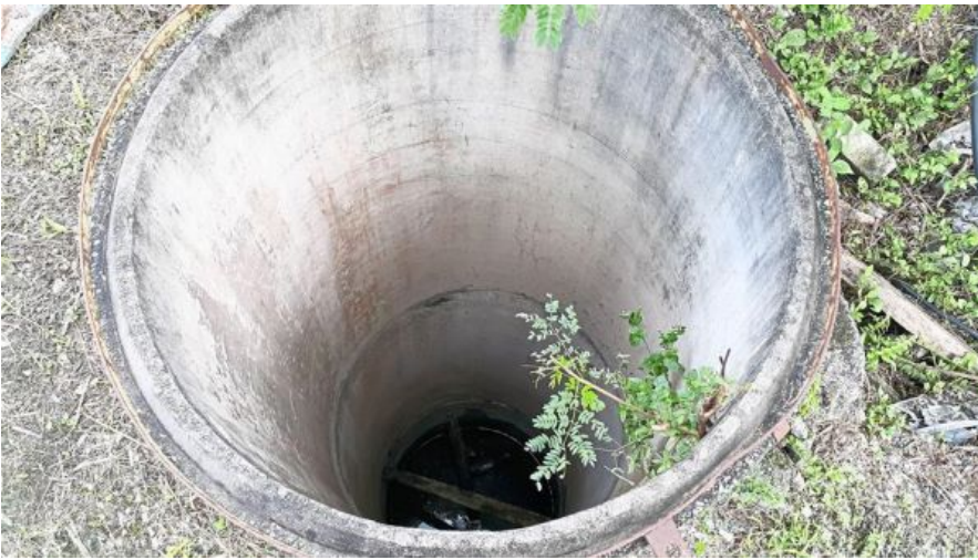
A concrete well believed to be used to collect water from Sungai Semenyih.
